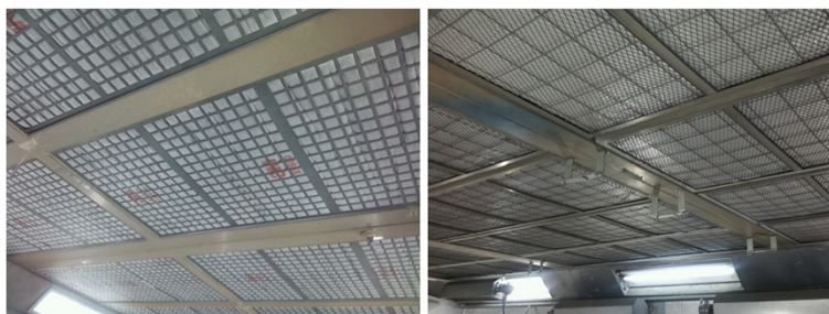
Figure 5 Ceiling inlet in the painting booth.
